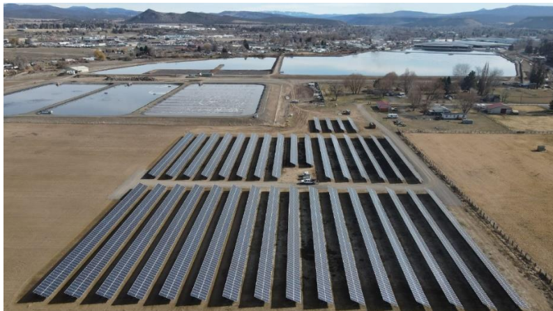
Solar field at the wastewater treatment plant facility.
