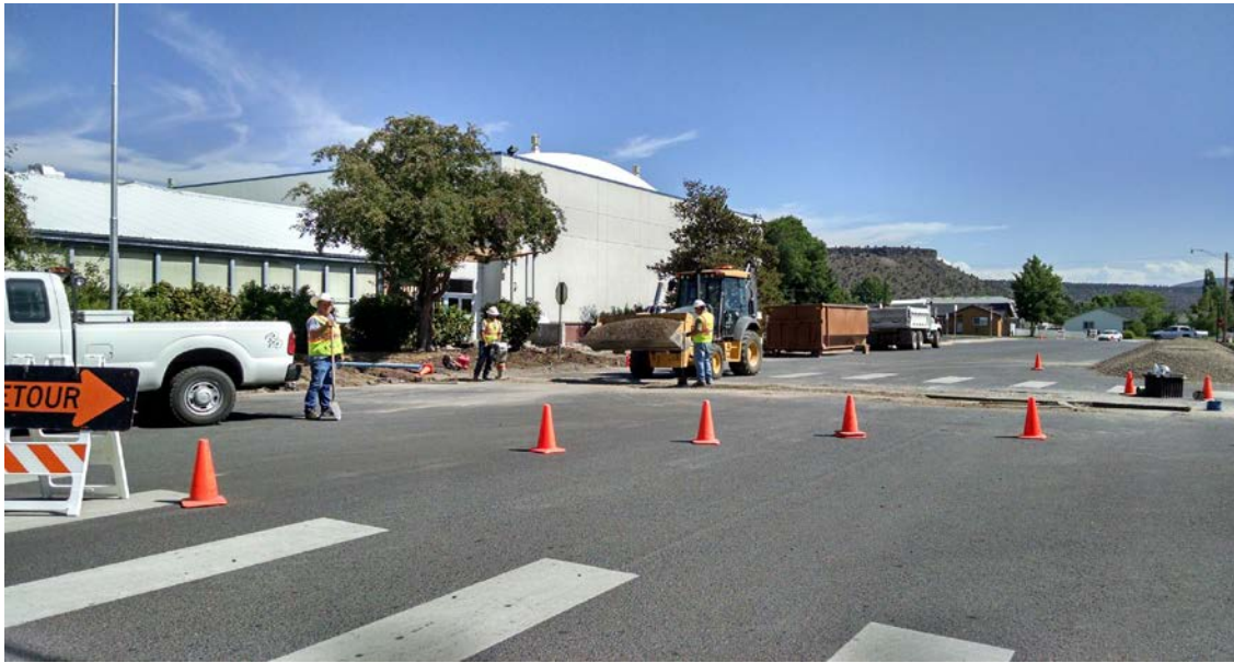
Members of the Water Department installing a new service to the middle school
