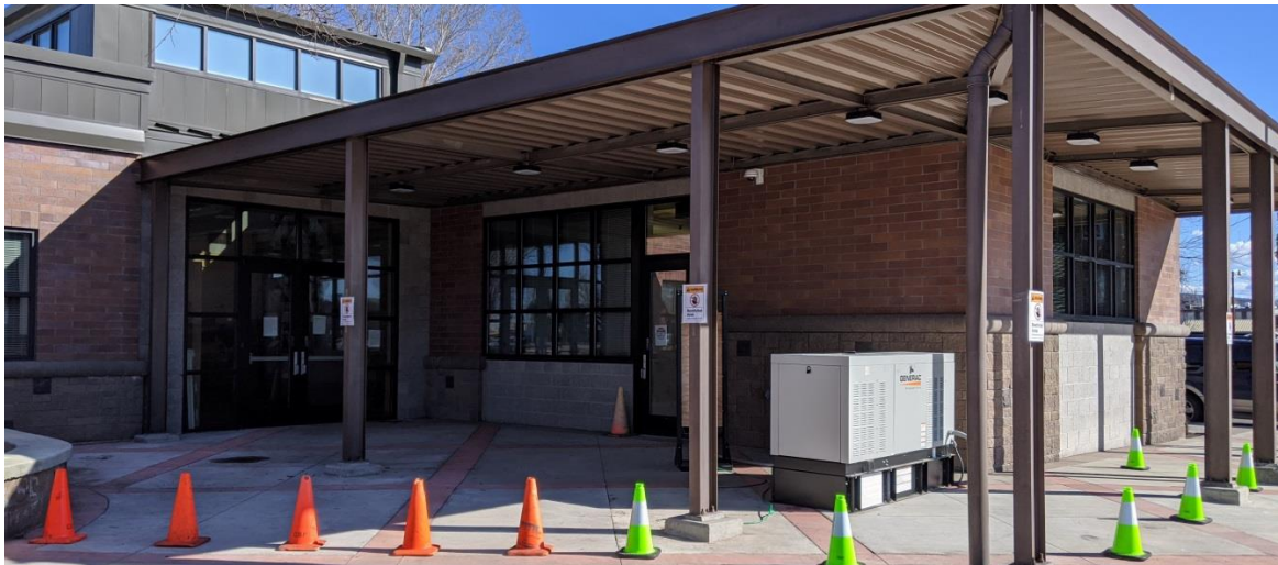
Backup generator needed for the dispatch center with the move to City Hall which was set up by IT.
