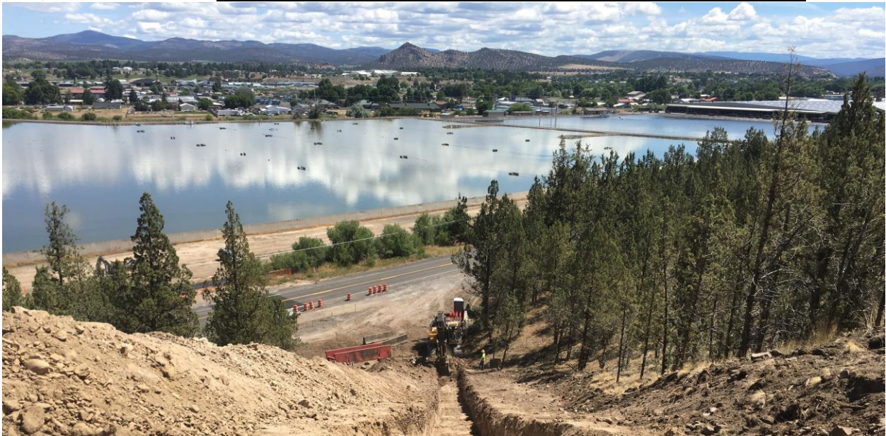
Beginning phase of the Airport Industrial Park Utility Expansion project- picture courtesy of Taylor NW
