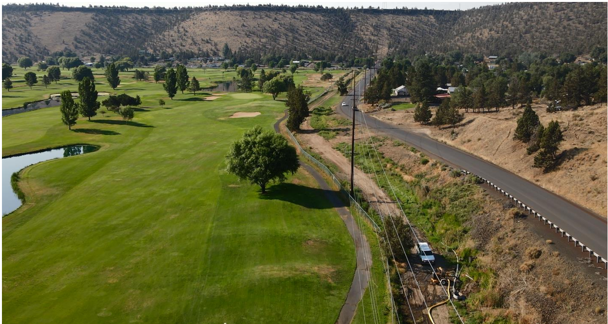
Work being done in August adjacent to the golf course to keep the People’s Irrigation ditch flowing for the summer.
