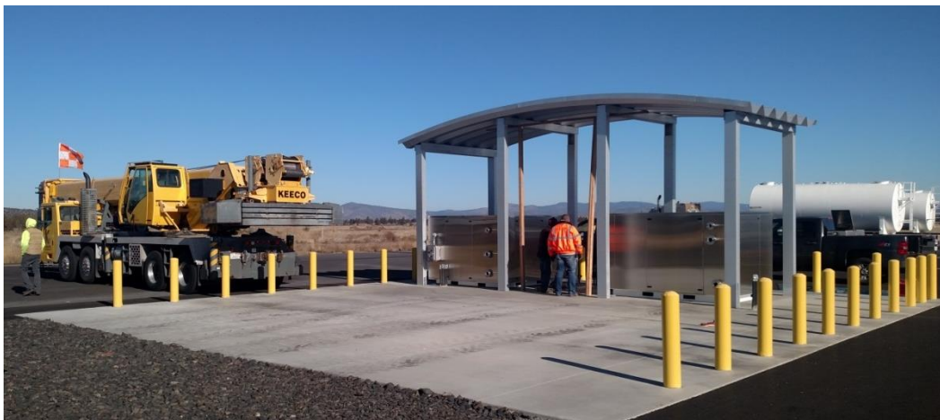
New fuel system, which is partially funded through a Connect Oregon grant, being installed at the airport during the first quarter.
